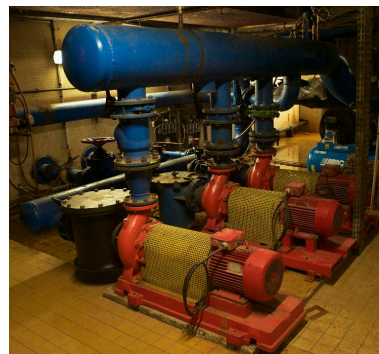
Pompes de filtration. Phot. Marie-Laure Monnehay-Vulliet IVR32_20170200266NUC2A
