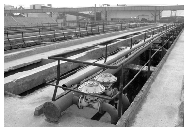
Stockage des pulpes. Phot. Francis Dubuc IVR22_19908000773Z
